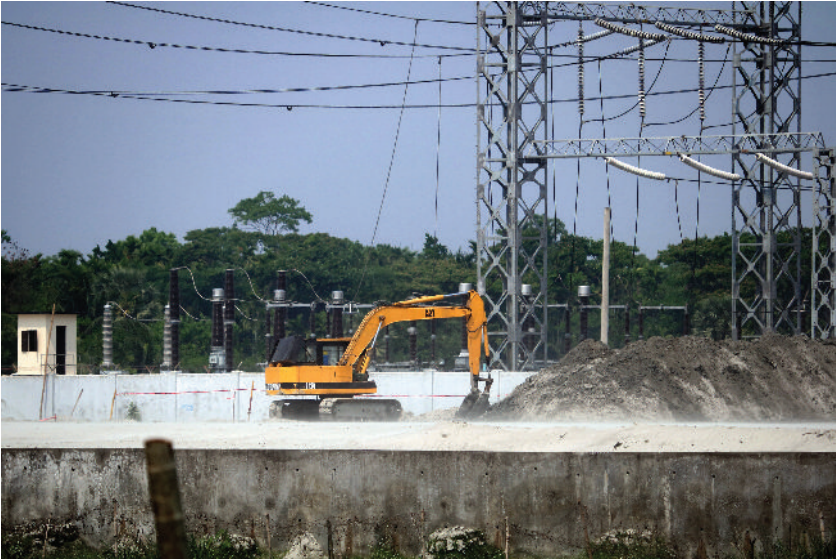
Photo 7: Construction site of Bhola IPP which is full of dust. Photo taken from other bank of Dehulia Khal. Photo: Hasan Mehedi
