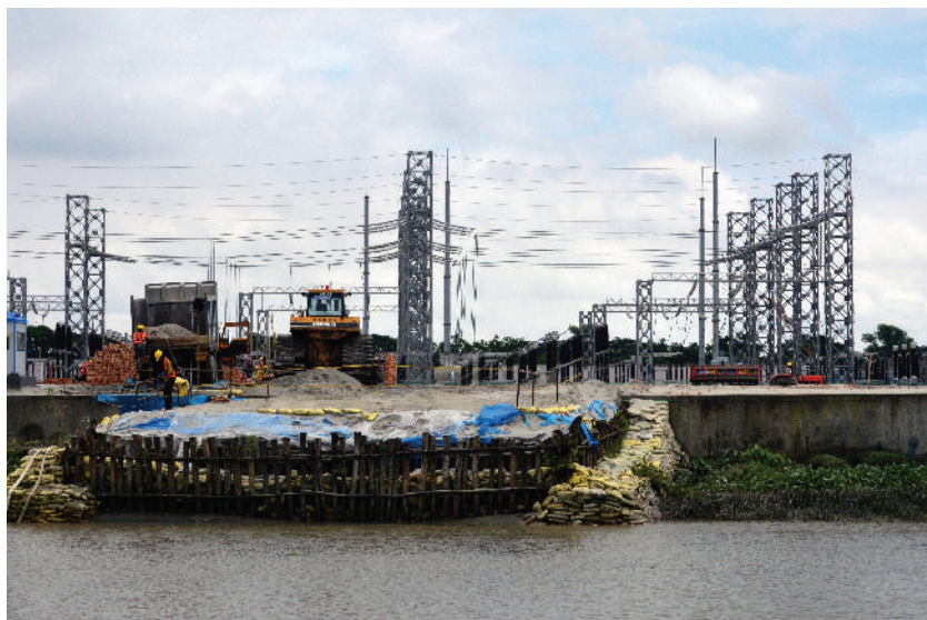
Photo 14: Different places of the Dehular Khal and Mandartoli Shakha Khal have been grabbed by the project executing agency. Photo: Mahbub Alam Prince
